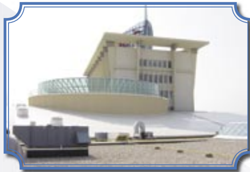
Exhaust vents, decorative fixtures and more. This is on the roof of Chinook Centre Shopping Mall
