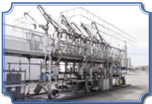
Industrial equipment and facilities
